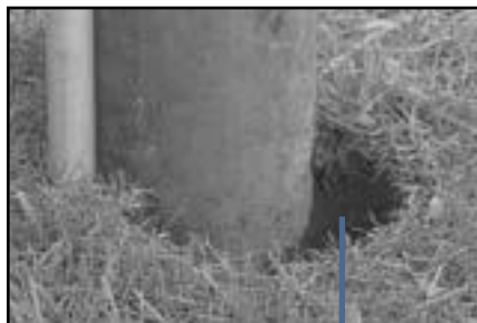
Faulty annular seal |
